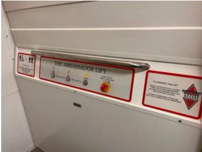
The lift control panel
