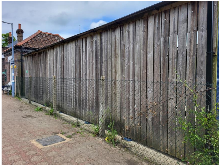
Above: Back of bike storage wall at Great Missenden station 11.2m x 2.84m
